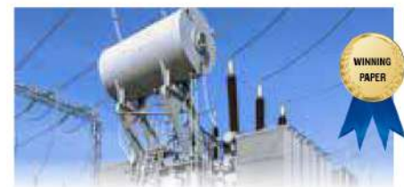
Enhancing the Sustainability/ Reliability: New Generation Natural Ester Based Transformer Oils
