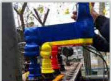
Substation Insulation Transformer Insulation
